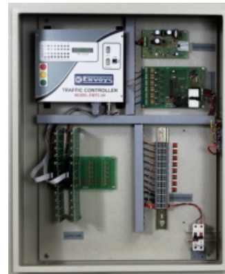
Inside View Of Controller Cabinet
